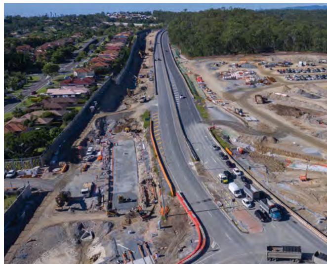
THE FUTURE PARKWOOD STATION AND PARK 'N' RIDE AT THE SMITH STREET AND NAPPER ROAD INTERSECTION.
